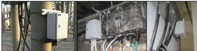
DAQ at Xincheng Substation
